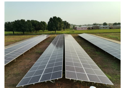
Mali: Rural Electrification
